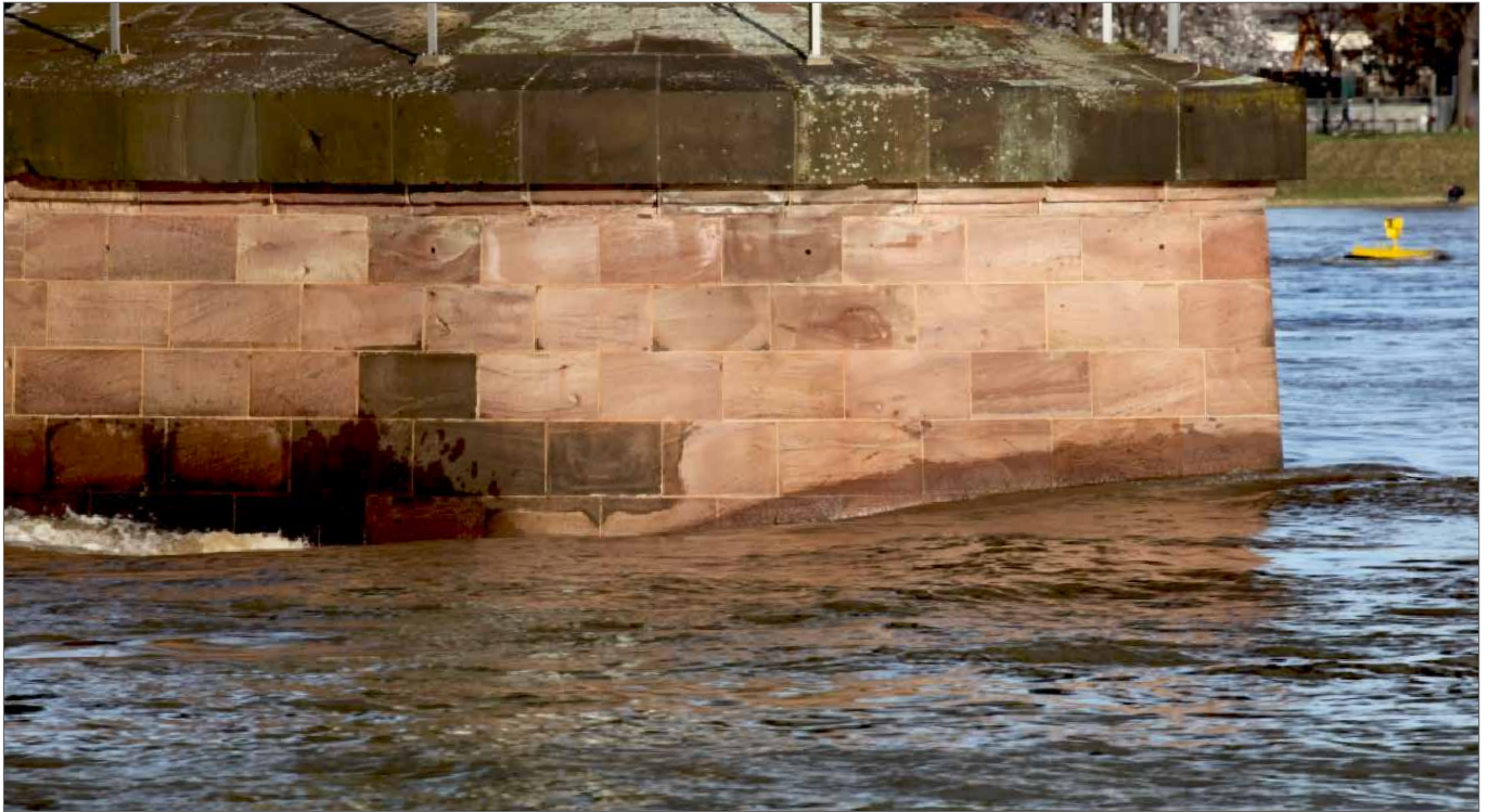
Fig. 3.4-1: Backwater effect at a pier of the Cologne Südbrücke in the Rhine; direction of flow from right to left [Waterways and Shipping Office Cologne]
